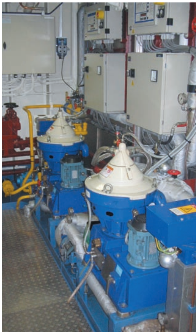
Two SA 815 separators installed onboard the Catharina KW145.
