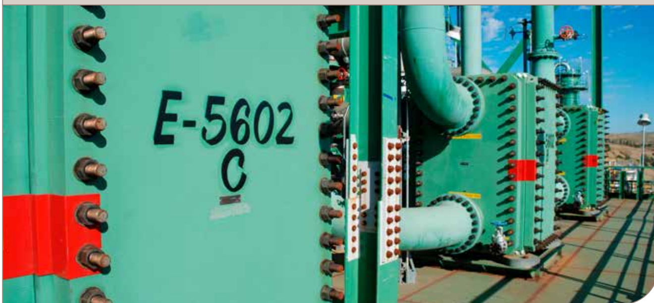
Three Compabloc CPX 120 heat exchangers ensure environmental compliance in a BELCO® flue gas scrubber. PHOTO: Jim Hill.
