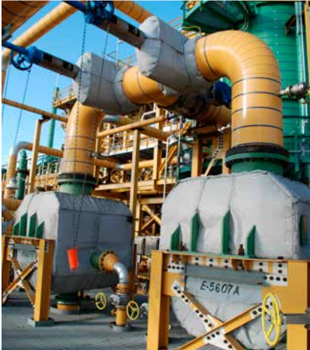
Two compact CPX 120 reboilers efficiently add heat to a CANSOLV® lean amine stripping tower. PHOTO: Jim Hill.
