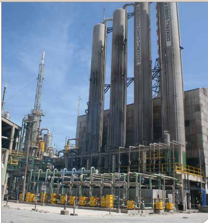
Thirteen Compablocs used as nitric acid coolers at the Monomeros Nitric acid plant in Colombia.
