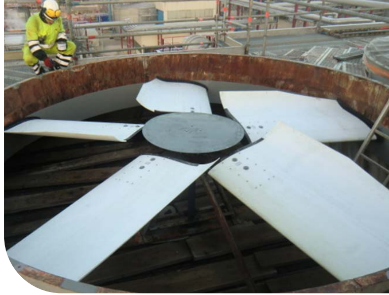
The new fan blades enabled a lower rotating speed, resulting in lower noise levels and reduced power consumption.
