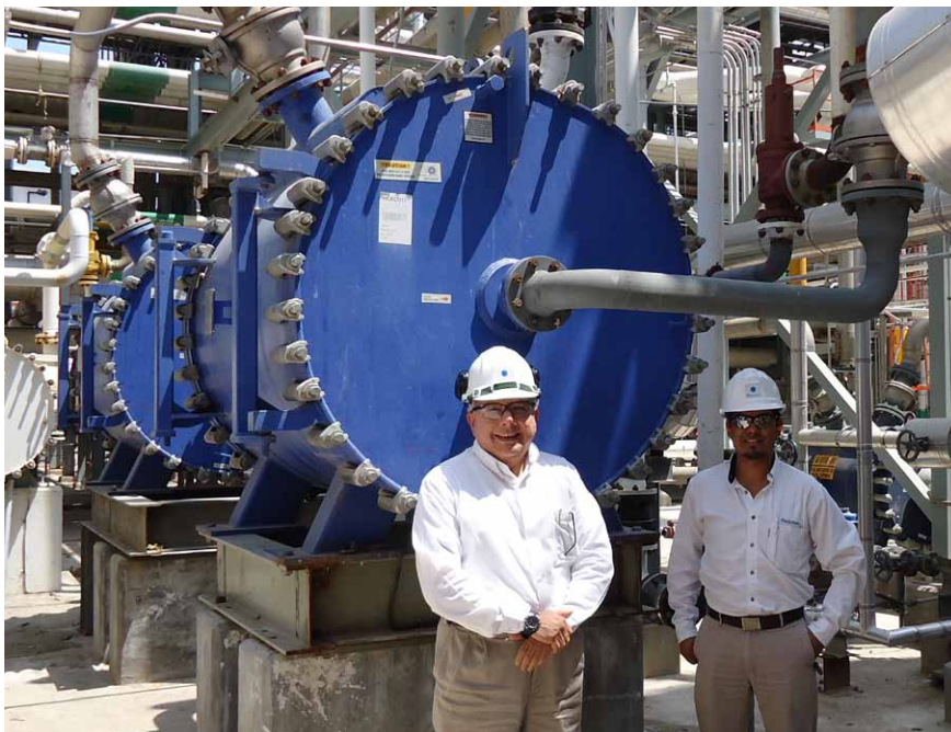
Miguel Angel Rivera Hernández, Engineering Manager and Armando Obregón, Project and Construction Quality Engineer at Mexichem, in front of two of the plant's spiral heat exchangers. "The performance is so good we hardly think about cleaning anymore", Armando Obregón says.
