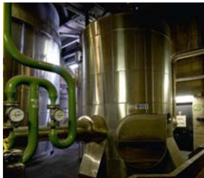
The flash vessel used in BASF's ammonium sulphate concentration process
