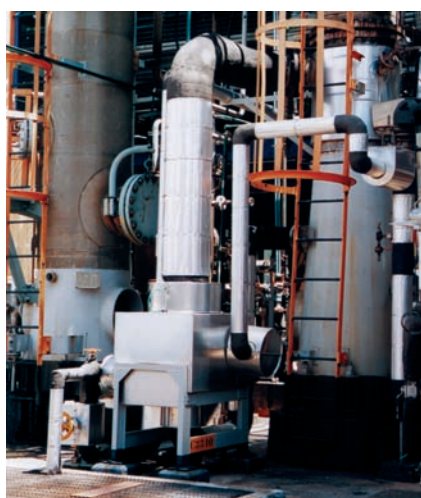
Compabloc installed as stripping column reboiler at an ethyl-acetate plant in Rhodia, Brazil
