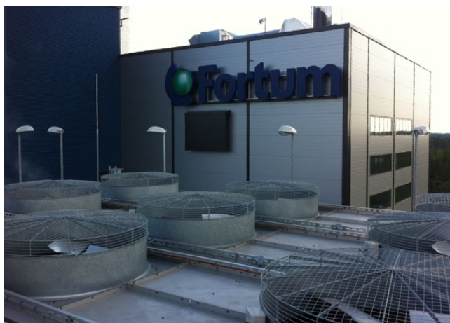
Alfa Laval FBLGS-1200-20-3A10 district heating liquid cooler
