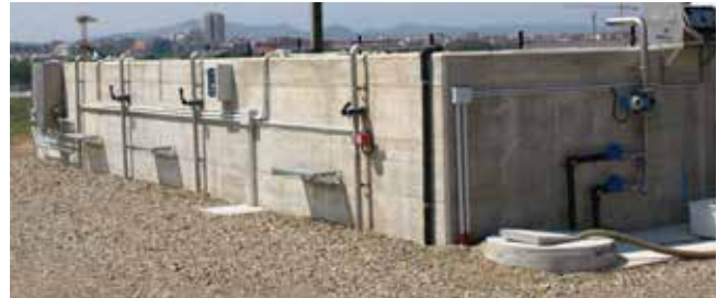
The membrane bioreactor plant at Viña Ijalba has a small footprint and can treat 40 m 3 /d wastewater per day.
