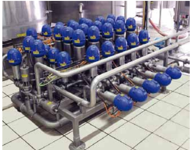
Moloko Dairy cream valve cluster with Alfa Laval Unique SSV, Unique Mixproof and LKB valves and ThinkTop valve sensing and control units.
