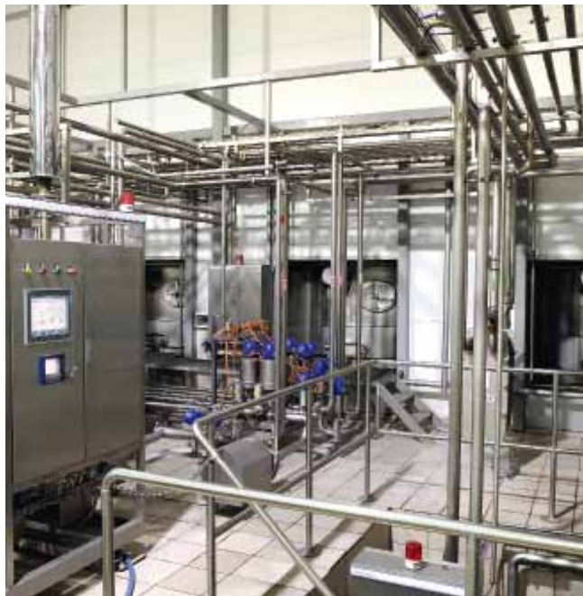
Moloko Dairy milk reception plant upgraded with Alfa Laval Unique SSV valves, LKB valves, ThinkTop valve sensing and control units, Solid C and LKH centrifugal pumps and energy-efficient agitators.
