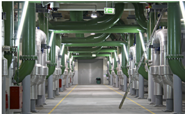
From the cooling plant, a pipe network provides the cooling for all the amenities – residential, commercial and sportive – for the entire man-made island of The Pearl Qatar.
