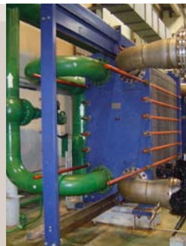
The Tianwan NPP uses a total of 46 gasketed plate heat exchangers from Alfa Laval.
