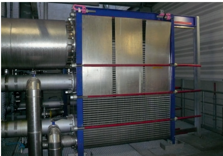
Two AlfaCond 800 units operate in parallel as purge condensers.
