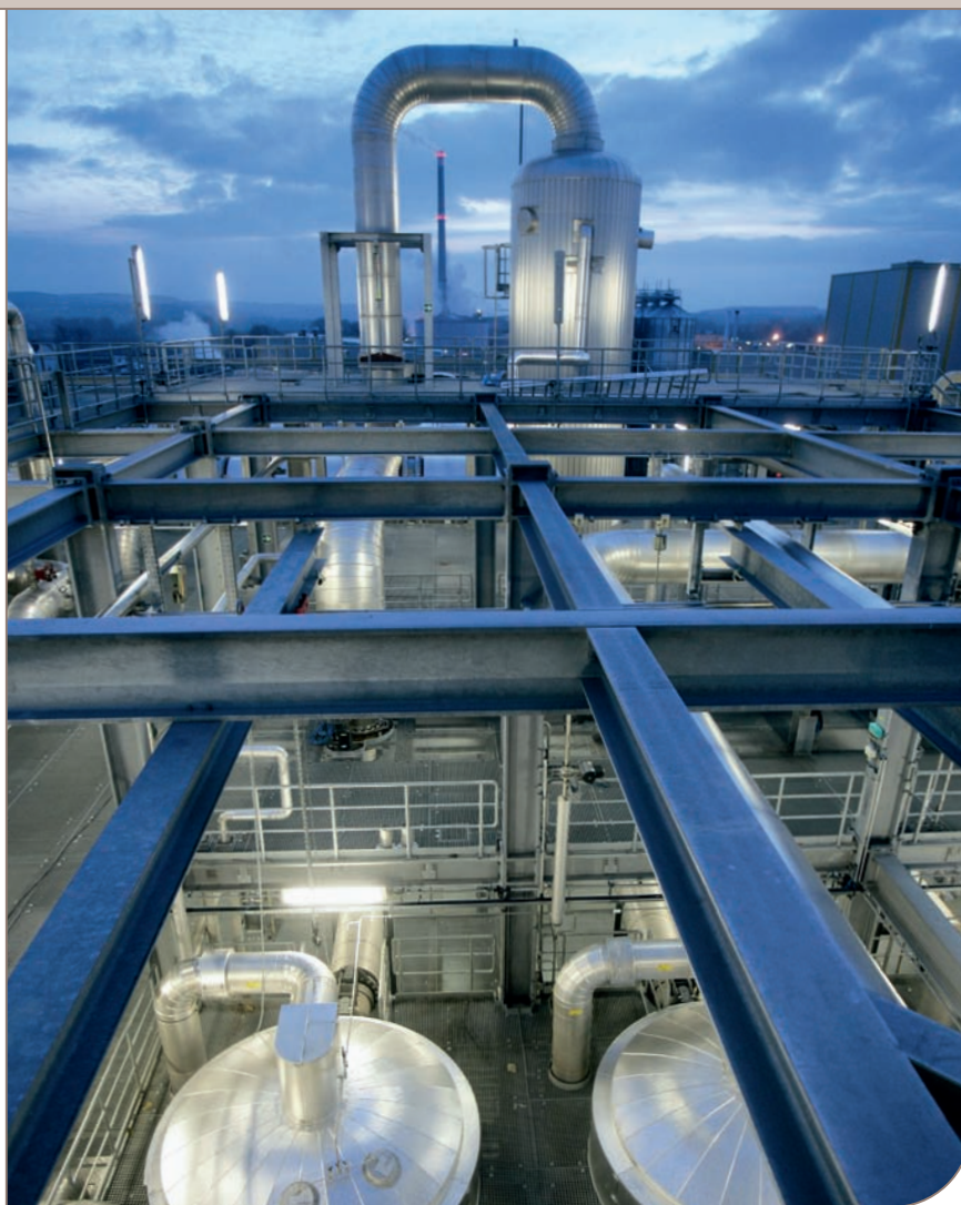
CropEnergies Bioethanol plant in Zeitz, Germany, currently has a total capacity of 360,000 m 3 of ethanol per year.
