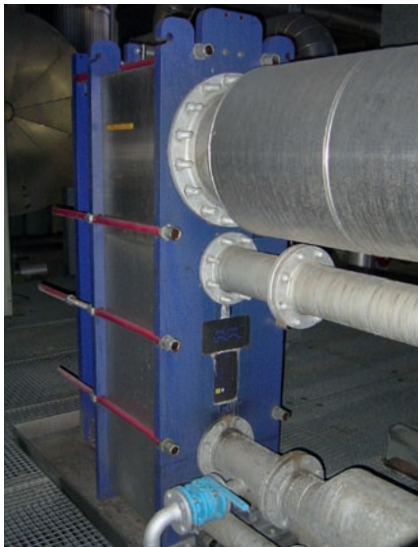
An AlfaCond 400 installed as a flash condenser for the evaporation system used in the production of DDGS.
