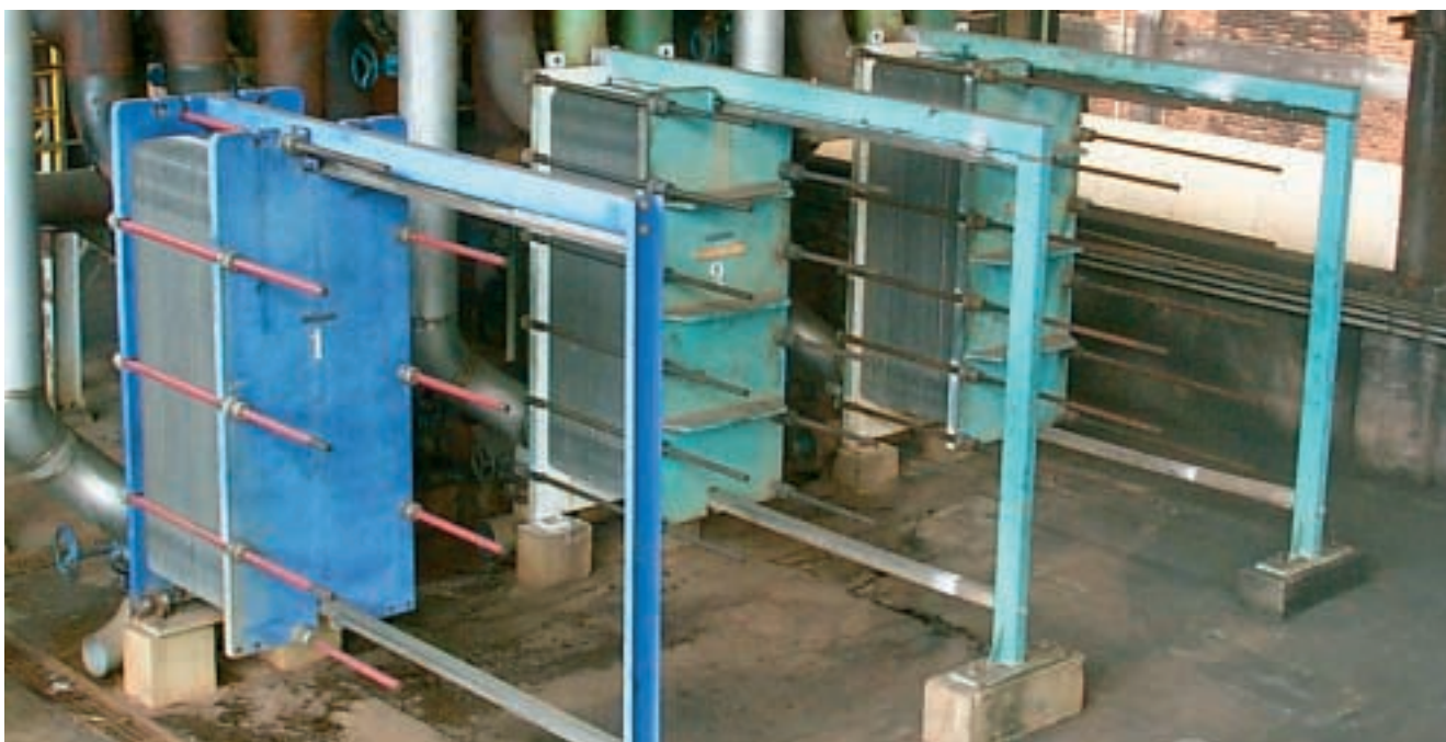
Replacing cooling coils with plate heat exchangers has increased yield and decreased maintenance costs
