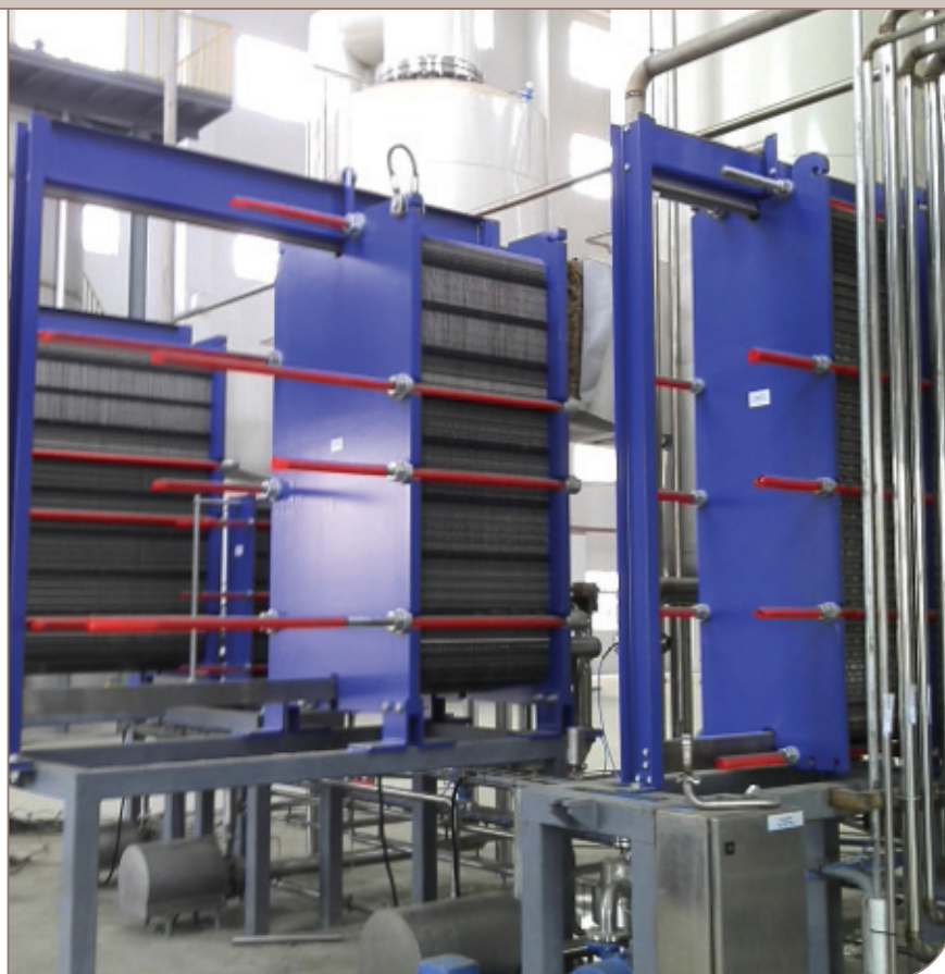
Two AlfaVap 500 evaporators and an AlfaCond 400 condenser installed at the Biok plant.
