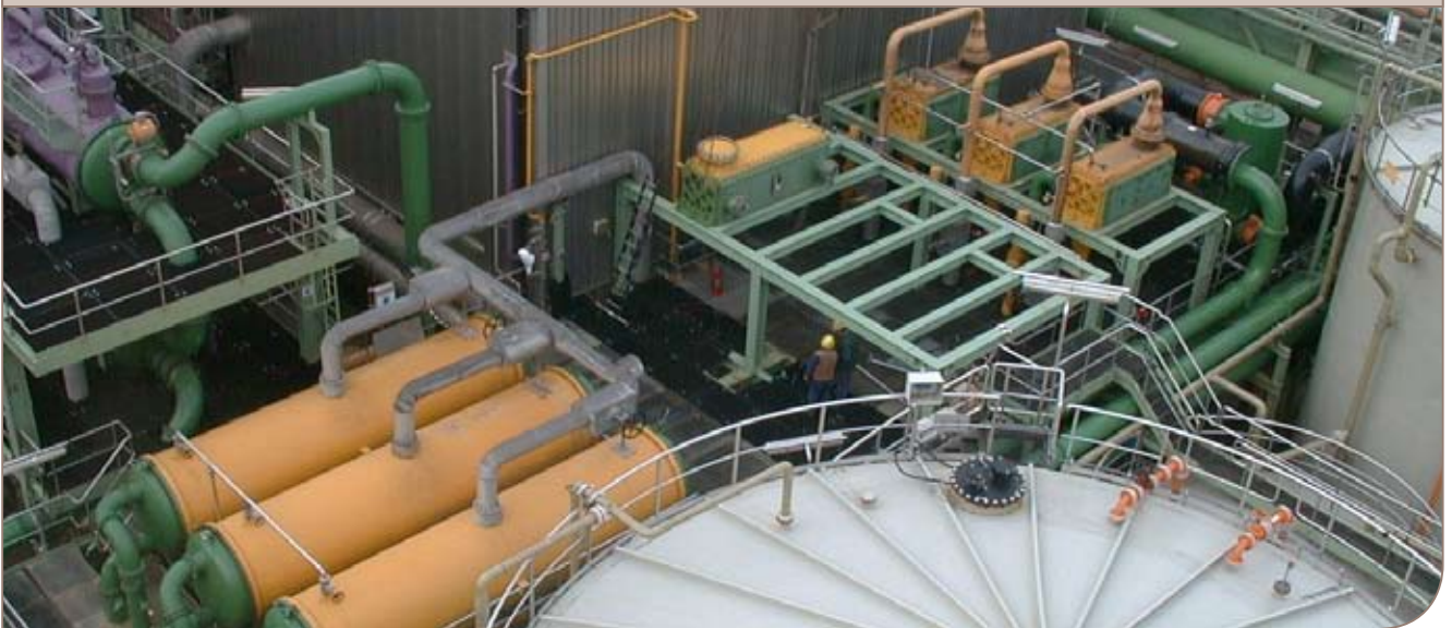
Three Compablocs (top right) with 50% higher capacity replaced three S&Ts (lower left) on half the footprint.
