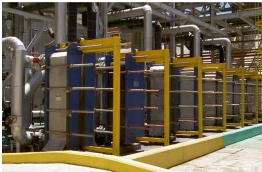
Six of the 16 heat exchangers at the Barrick Zaldivar copper mines in Chile. The mechanical construction of the Alfa Laval Plate heat exchangers makes them easy to open and clean by unscrewing the tightening bolts.
