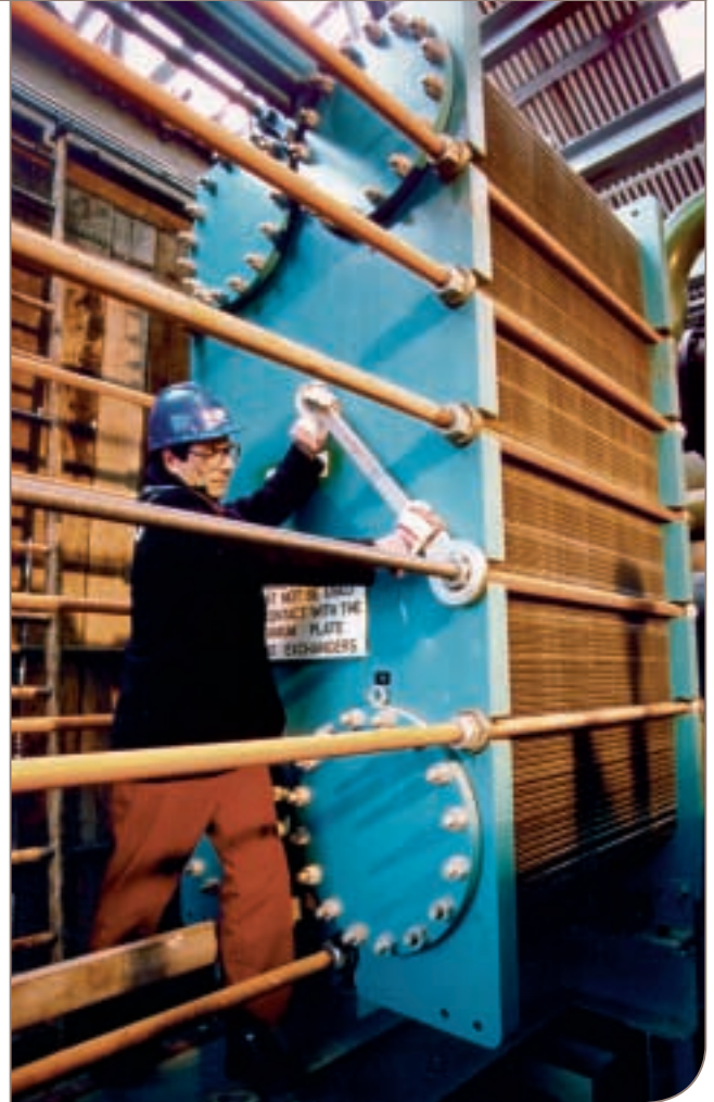
The plate heat exchanger ammonia still condenser installed at Brunner Mond in Northwich, UK.
