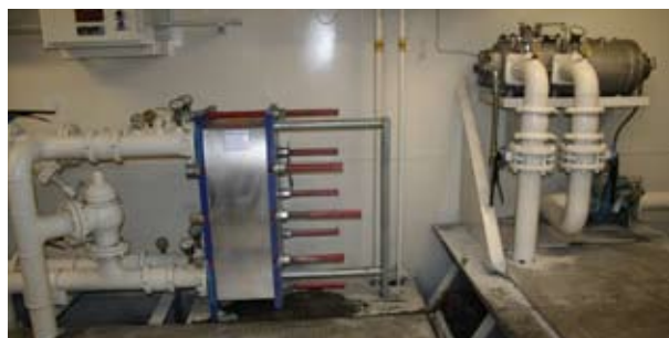
Plate Heat Exchanger and Eliminator
