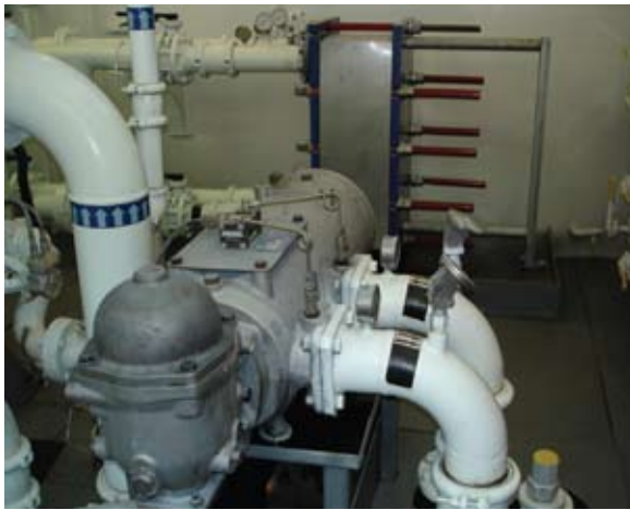
Eliminator filter and Plate Heat Exchanger
