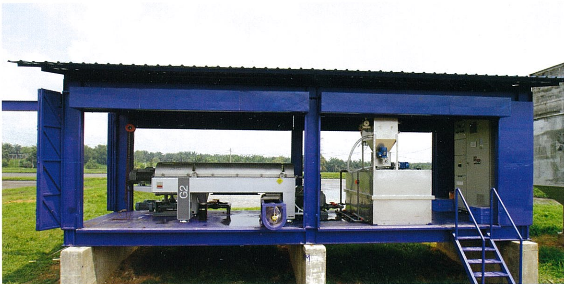
Decanter modular system installed for POME
