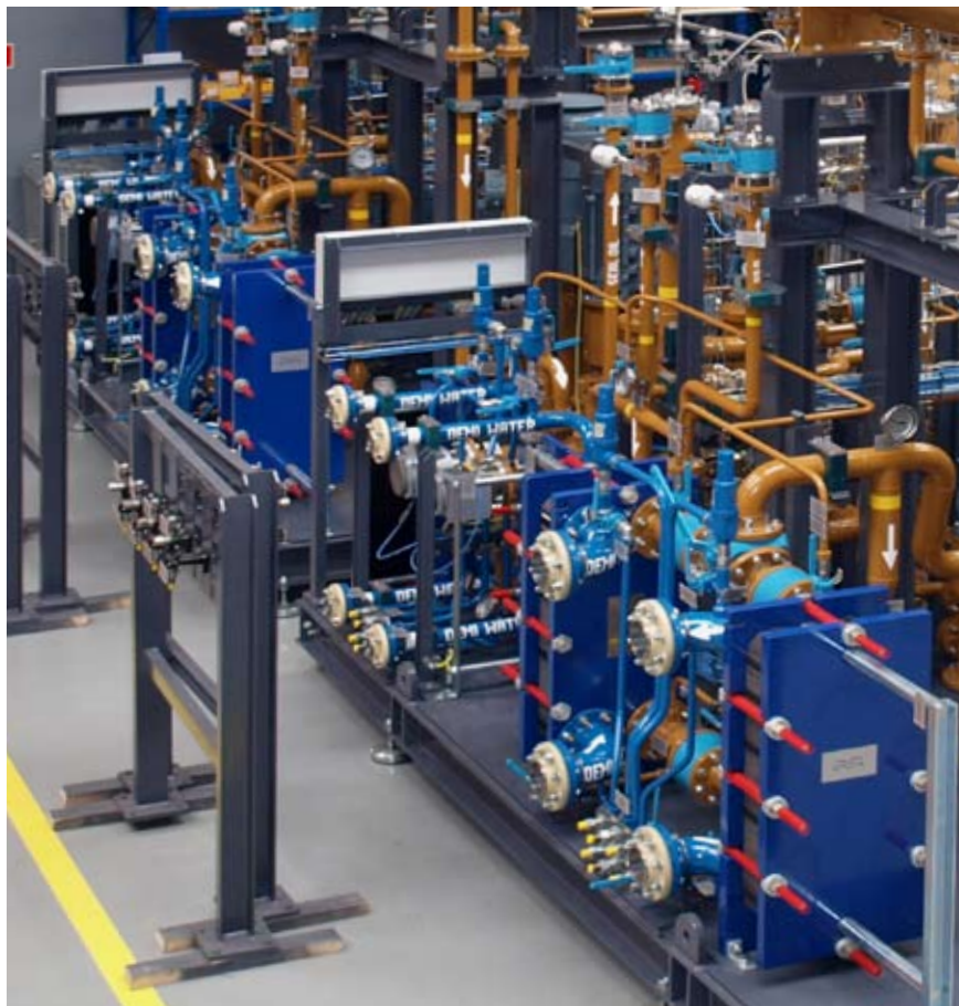
Alfa Laval plate heat exchangers installed for turbine cooling at the Medupi Power Station.
