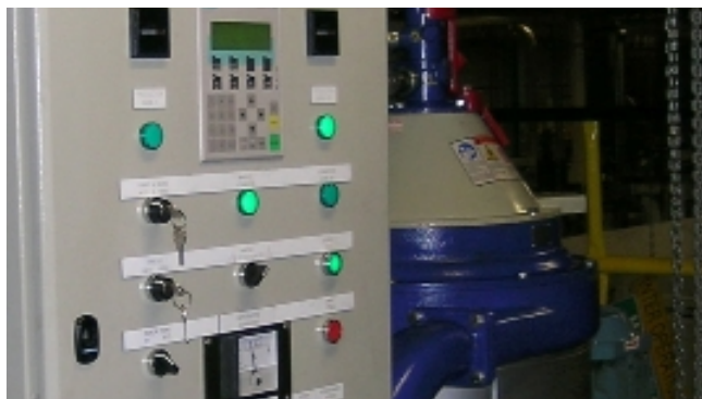
Alfa Laval high speed centrifugal separation system installed at Ford in Bordeaux to clean coolant.
