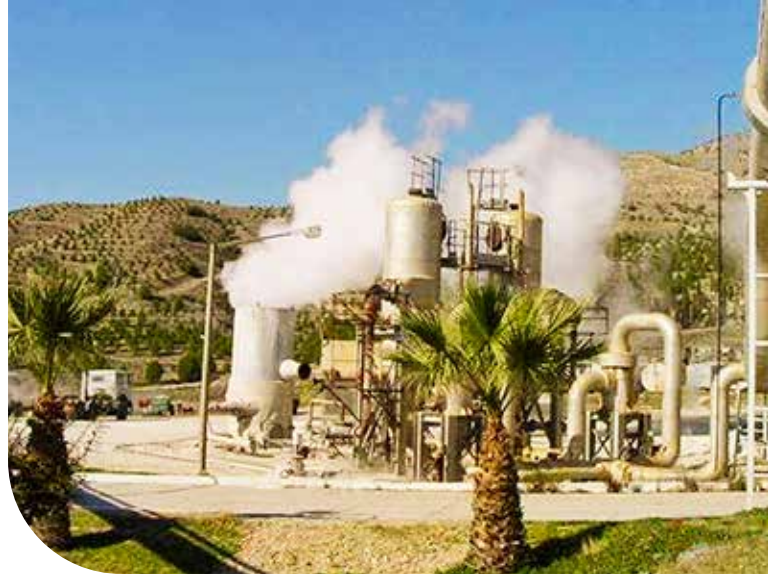
The Balcova project is an interesting "model project" distributing heat and domestic tap water to local households via a district heating network and with geothermal water as medium.
