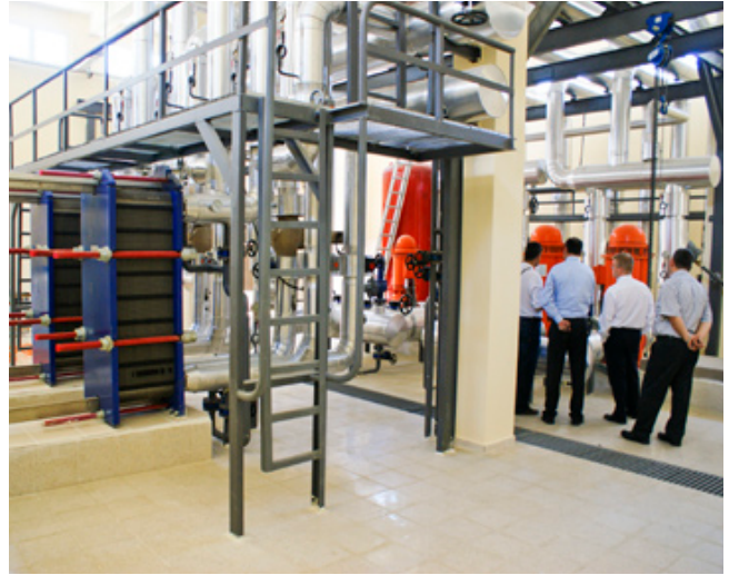
There are some 1500 PHEs from Alfa Laval at work within the network.
