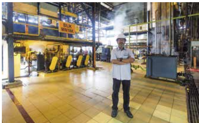
The oil room is the heart of a mill, where oil is extracted from raw material.
