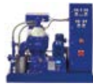
Fuel and lube oil cleaning
