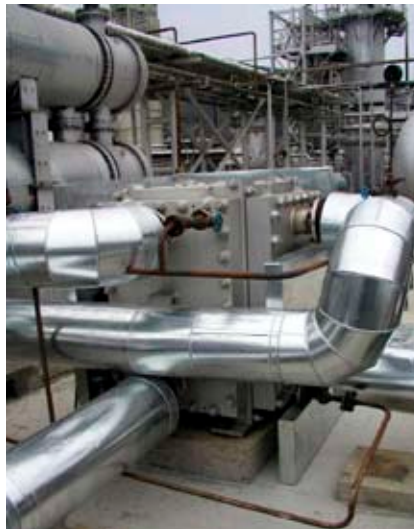
One Compabloc preheating crude since 2002 in a Russian refinery.
