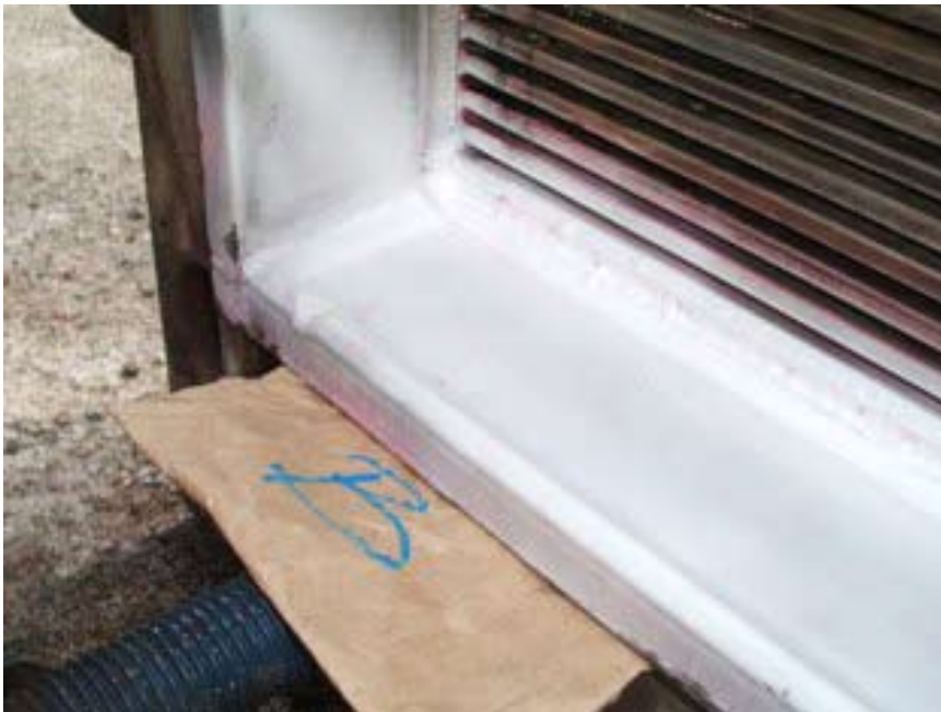
Here the result of the dye-penetrant test after a corner weld has been TIG repaired.
