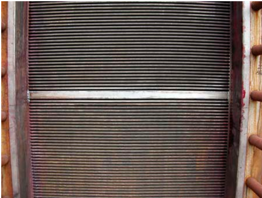
Photo showing a cross-leaking Compabloc channel sealed with a metal-strip.
