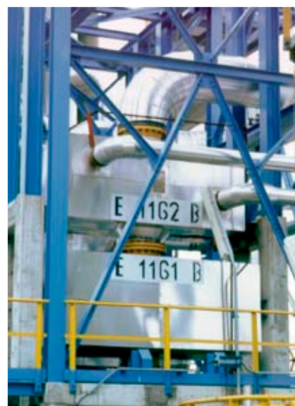
Two out of four Compablocs operating since 1997 as ADU overhead vapour condensers in a European refinery.
