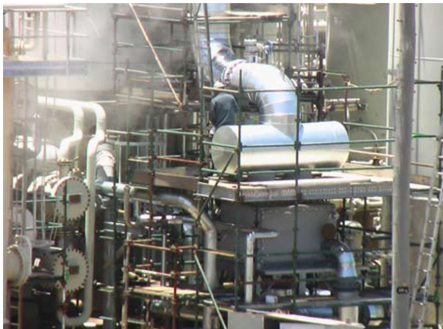
One Compabloc operating since 2006 as naphtha reboiler in an Australian refinery.
