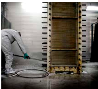
This means the hydro-jet passes through the heat exchanger when the nozzle is tilted in 45 degree angle.
