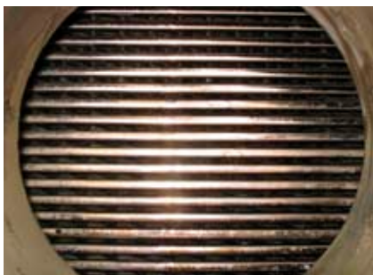
Endoscopic photo of hot stripped water circuit taken from the inlet nozzle of a Compabloc operating since 2003 as interchanger in a SWS unit in a South America refinery. Photo shows before and after chemical cleaning.
