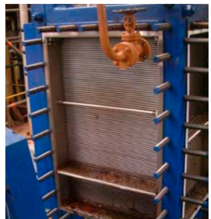
Photo showing before and after high-pressure water-jet cleaning of the cooling water circuit of a Compabloc operating as condenser in the solvent recovery part of a paraffin removal plant in Europe.
