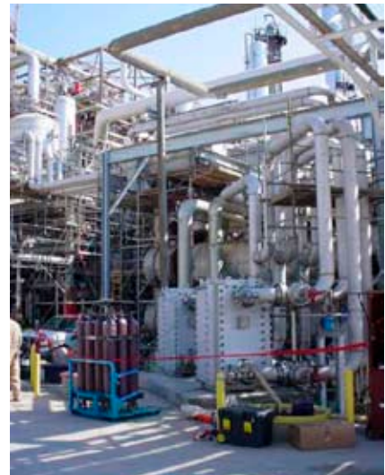
Two Compablocss preheating crude since 2004 in a North American refinery.
