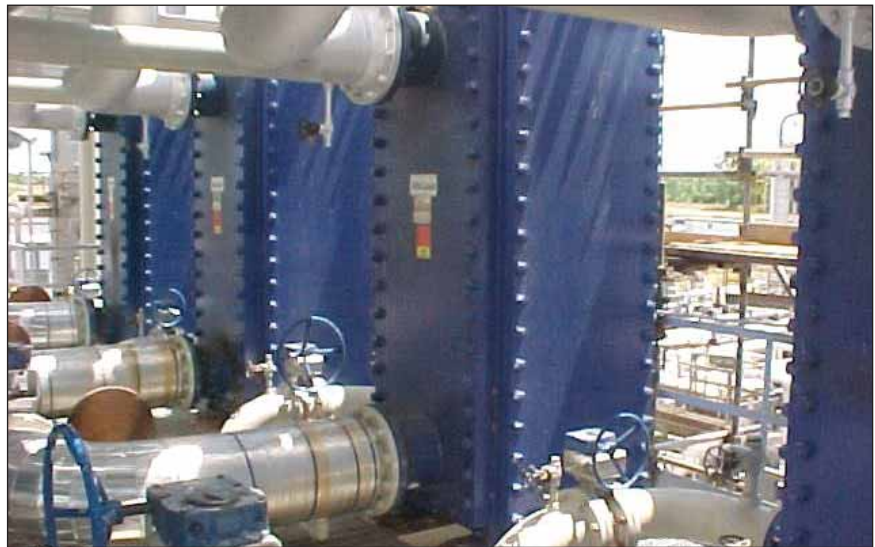
Figure 8 CPHE installation for recovery of a total of 14 MW from FCC overhead vapours into BFW loop.
