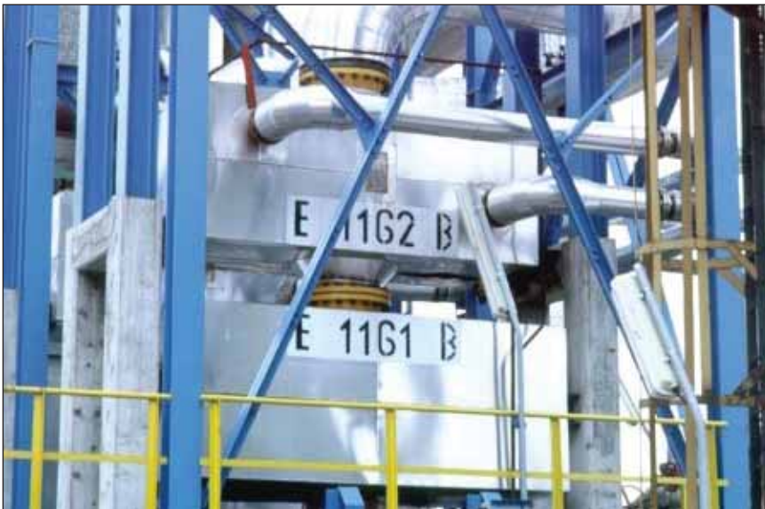
Figure 6 One of the two CPHE pairs mounted on top of each other for preheating BFW and crude by means of naphtha toppings
