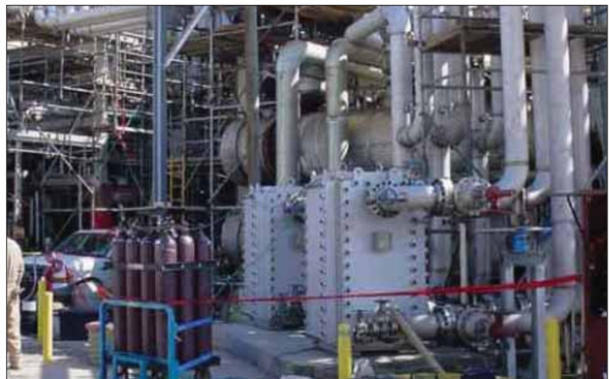
Figure 5 Two CPHEs used for crude preheating by means of HVGO
