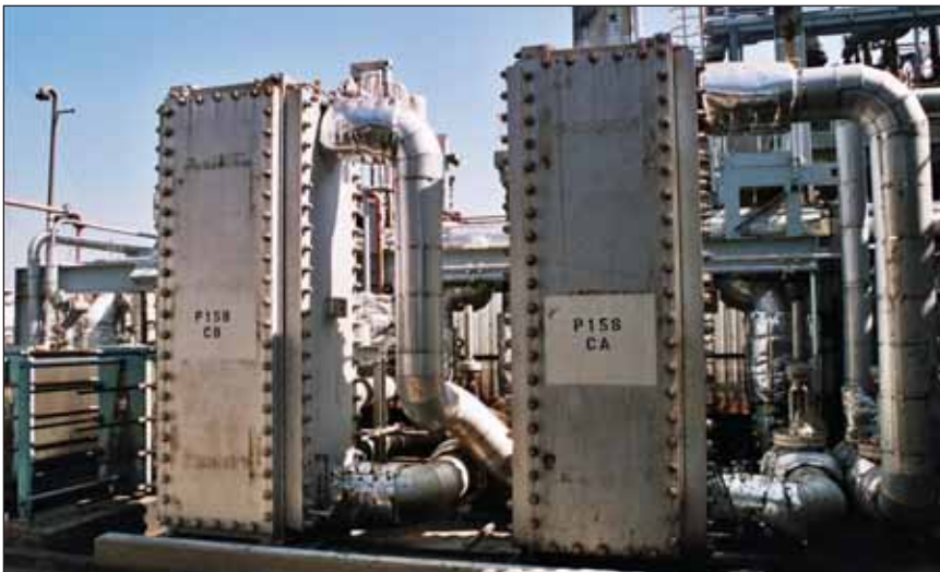
Figure 7 Heat-recovery installation in UK, preheating BFW by means of atmospheric residue
